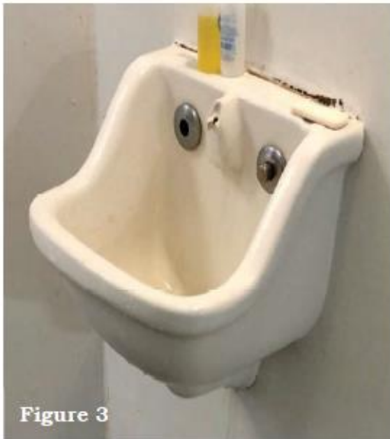
Detainee Cell Sink with Missing Hot Water Button
